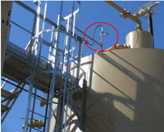
IS-20-VR installed on salt water disposal system tank
